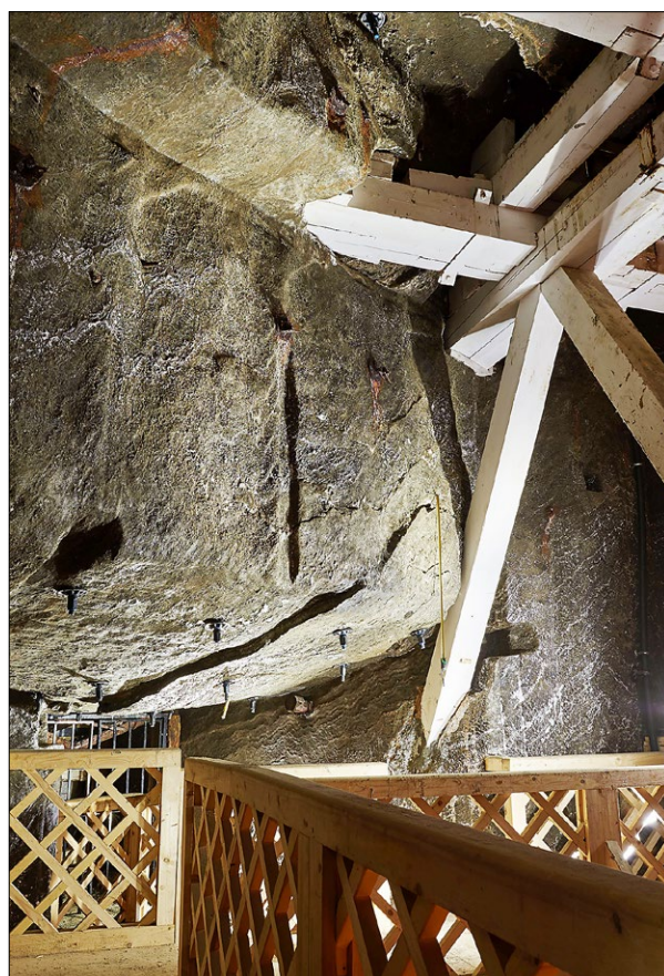
Fig. 3. Wieliczka Salt Mine—reconstruction of truss support in the “Gołuchowski” cavern, using modern anchoring support; photo by AMC.
