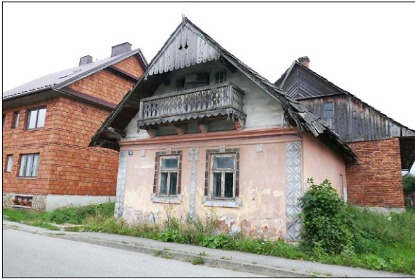
Fig. 4. Abandoned masonry house from 1900, located Jana III Sobieskiego Street, entered into the monuments records, record No. 237/1179; photo by A. Korzeniowska.
